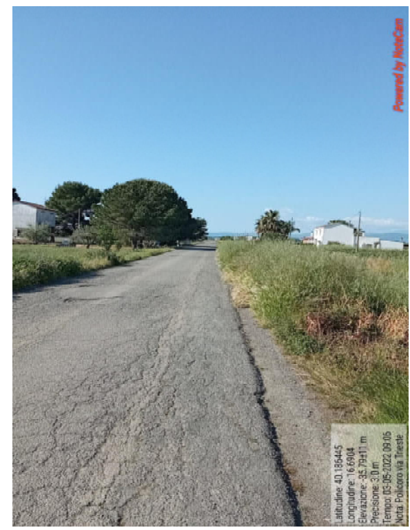
Int.6.3.7.1 Via Trieste Decesp. scarpate stradali
