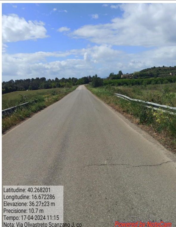
Int.6.3.3.1 Via Olivastroto Decesp. scarpate stradali
