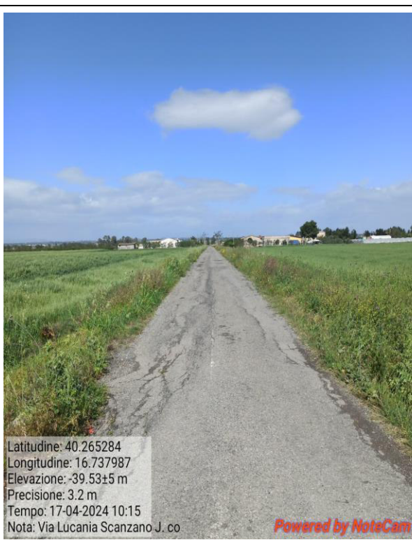
Int. 6.3.15.1 Via Lucania Decesp. scarpate stradali
